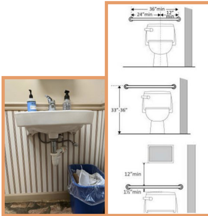
Rear grab bar should meet designated requirements.
