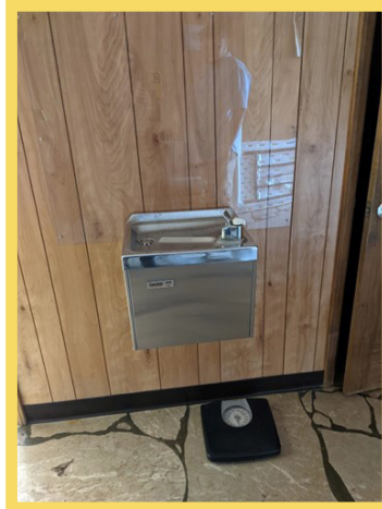
Fountain does not meet current design standards.
