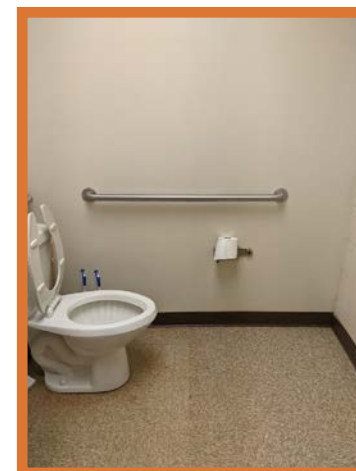
Toilet paper dispenser needs to be closer to the toilet.
