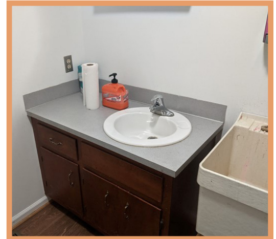
Not enough knee space under the sink
