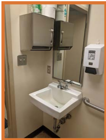
Pipes should be insulated
