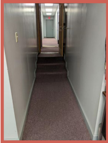
There are currently steps throughout Town Hall and no accessible route around them.
