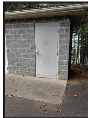
Slope is too steep to safely access the restroom from accessible space.
