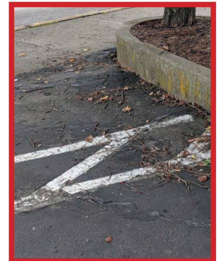
Access aisle is unlevel.
