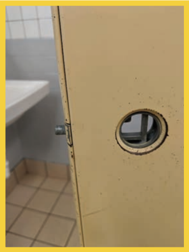
Recommend replacing damaged lock.
