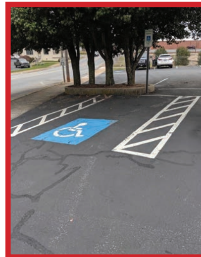
Access aisle needs to be 5 ft. wide.
