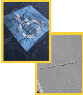
Seal cracks exceeding 1/2 inch.
