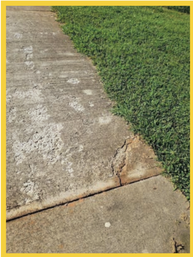
Cracks exceeding 1/2" must be sealed.
