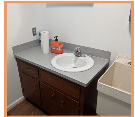
Not enough knee space under the sink
