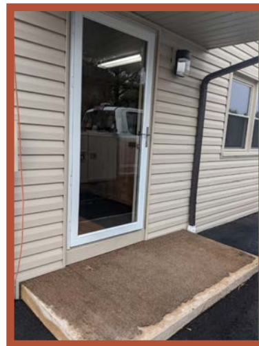
Entrance should be flush
