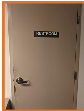
Signage should be in Braille and mounted on the latch side of the door at regulation height.
