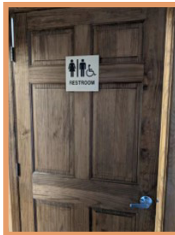
Accessible restroom signage should be placed on the latch side of the doorway.
