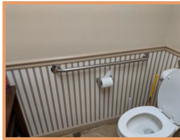
Side bar grab needs to meet designated requirements.
