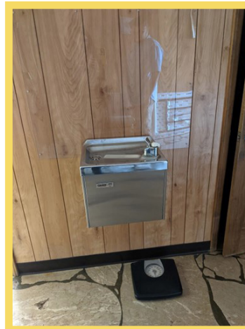
Fountain does not meet current design standards.
