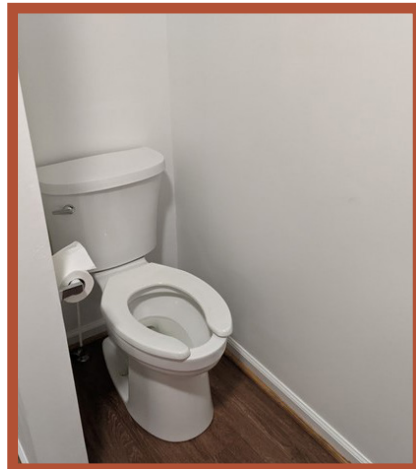
There is currently not enough clearance around the toilet
