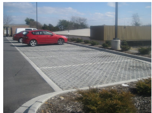
Pervious pavement helps control stormwater runoff
